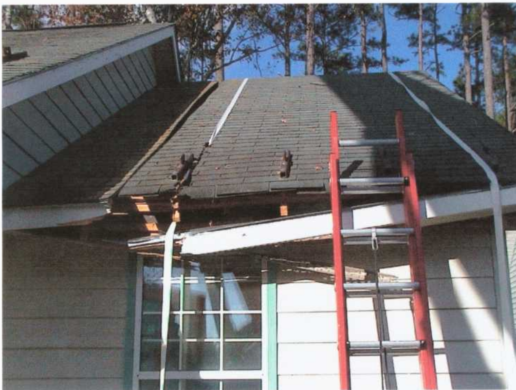
Figure 5. Roof of 3656 Eagle Trace with Orage Corporation Straps After Testing.
